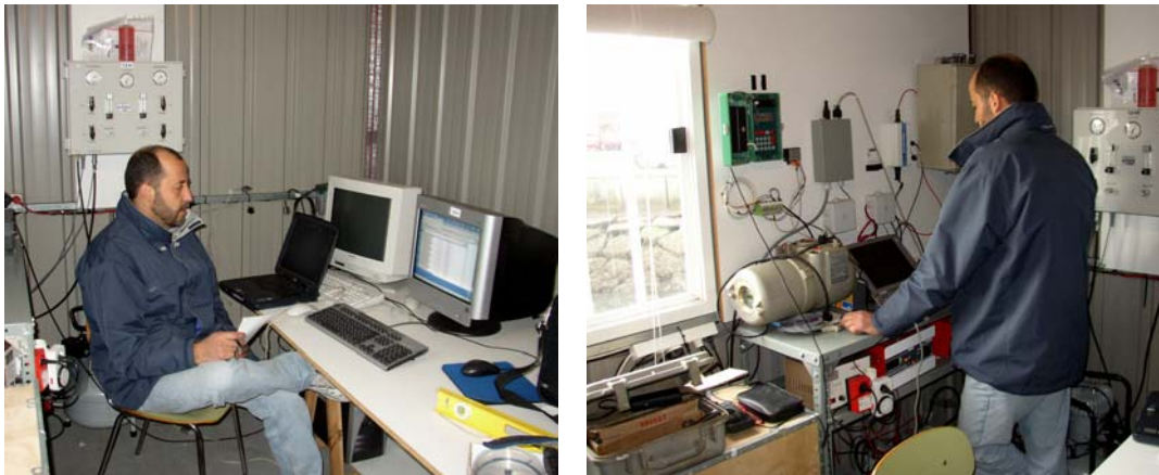
Figure 11 Interior of the hut with the computers and the rest of the electronic devices for the tide gauges.
