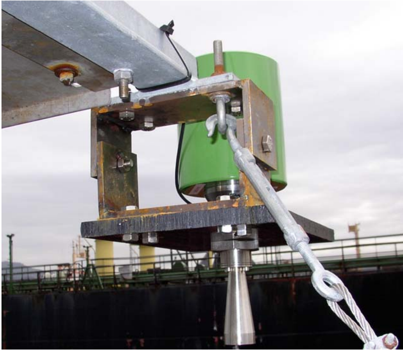
Figure 7 Horn antenna of the SEBA tide gauge.
