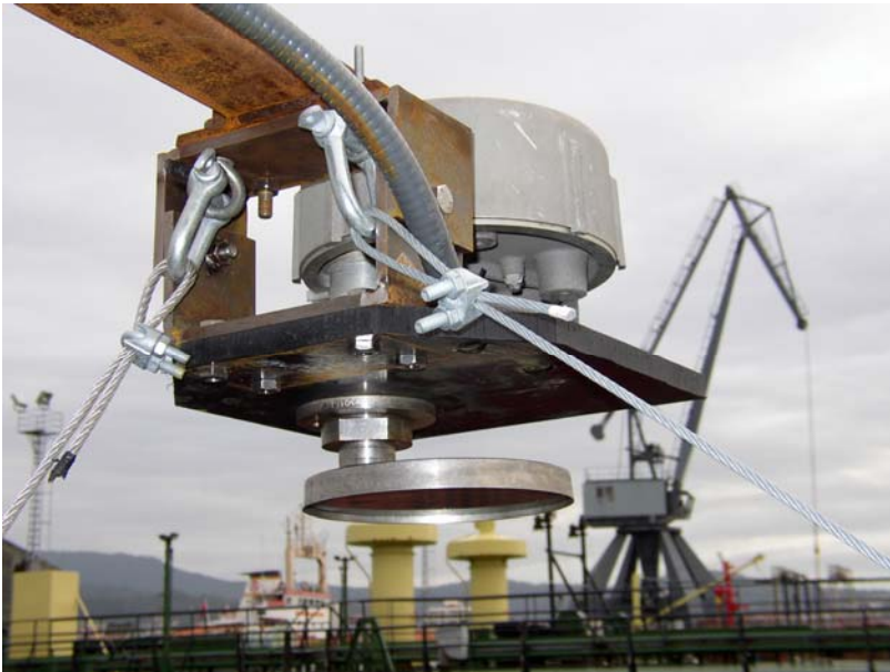
Figure 5 Horn antenna of the RADAC tide gauge.
